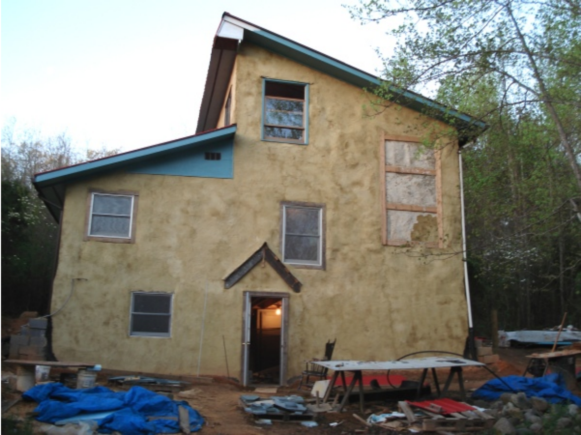
The Little Flower straw bale house under construction; photo taken in 2006 by Roger Straw.
